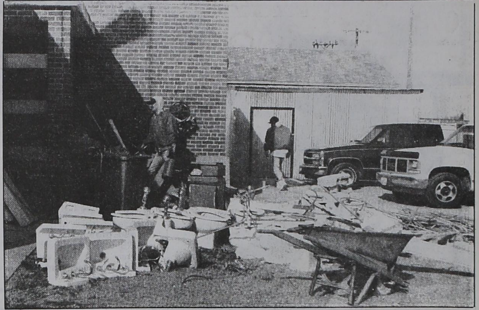
TAKING SOME OUT AND PUTTING SOME IN —Remodeling work at Plains Memorial Hospital is underway in the east wing of the hospital, which is being converted to a geriatrics psychiatric unit. If the
