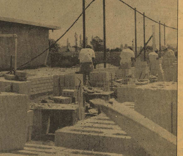
CONSTRUCTION is well underway on the addition of classrooms to South Grade School. Contractors have completed the walls of the new cafeteria for the Grade Schools. Classrooms and cafeteria should be ready for occupancy in the fall. —Staff Photo
