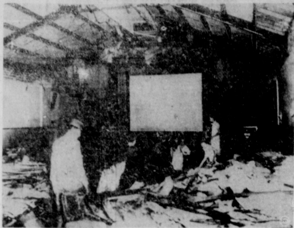
The acoustic ceiling of a Houma, Louisiana, theater, built last October, crashed without warning on a startled audience of 100 persons. At least 40 persons were injured, some of them seriously. (NEA Telephoto).
