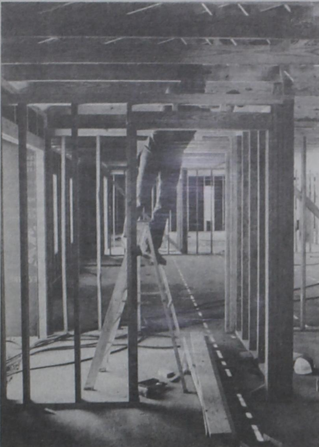
AMID A MAZE of wall studs and ceiling joists, Dudley Conner of Richardson Construction Co., Littlefield, measures for a door header in the new government office building being constructed at Southwest Second and Belsher. The building will house the ASCS, Soil Conservation Service and Farmers Home Administration offices.
