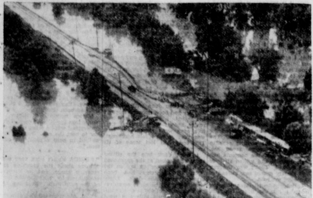
MEN AND FLOOD WATERS —Workmen near an almost break in the road, struggle to keep highway 4 open between St. Louis and St. Charles, Missouri. The riproaring Mississippi and her little sister, the Missouri, have knocked out 71 highways between Kansas City and St. Louis. (NEA Tele photo).
