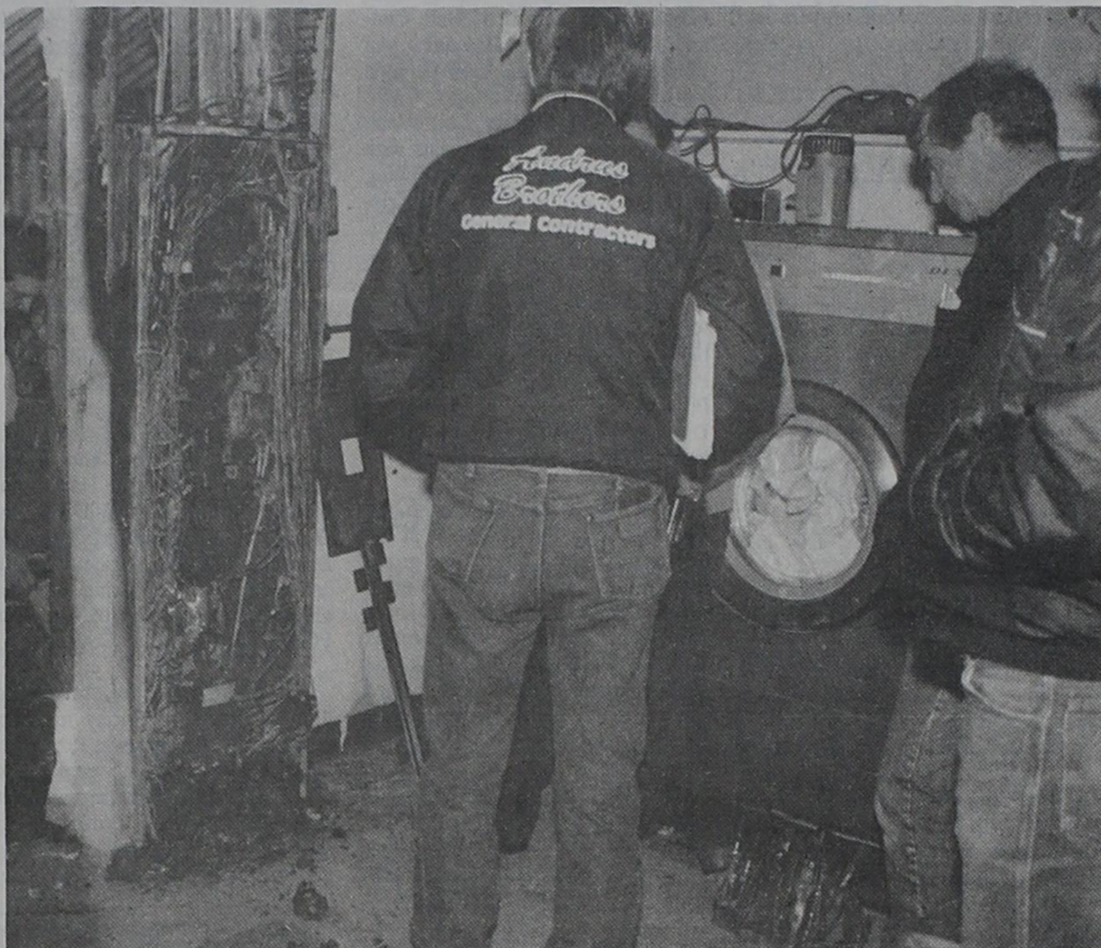
WHERE IT ALL STARTED—Contractors look at the damage to the main electrical switch panel in the laundry area of Canterbury Villa Nursing Home in Dimmitt Monday. The panel and a portion of the wall beside it were damaged by a fire Saturday morning, which caused the evacuation of the home's 71 residents, none of whom were injured in the fire. Photo by Linda Maxwell
