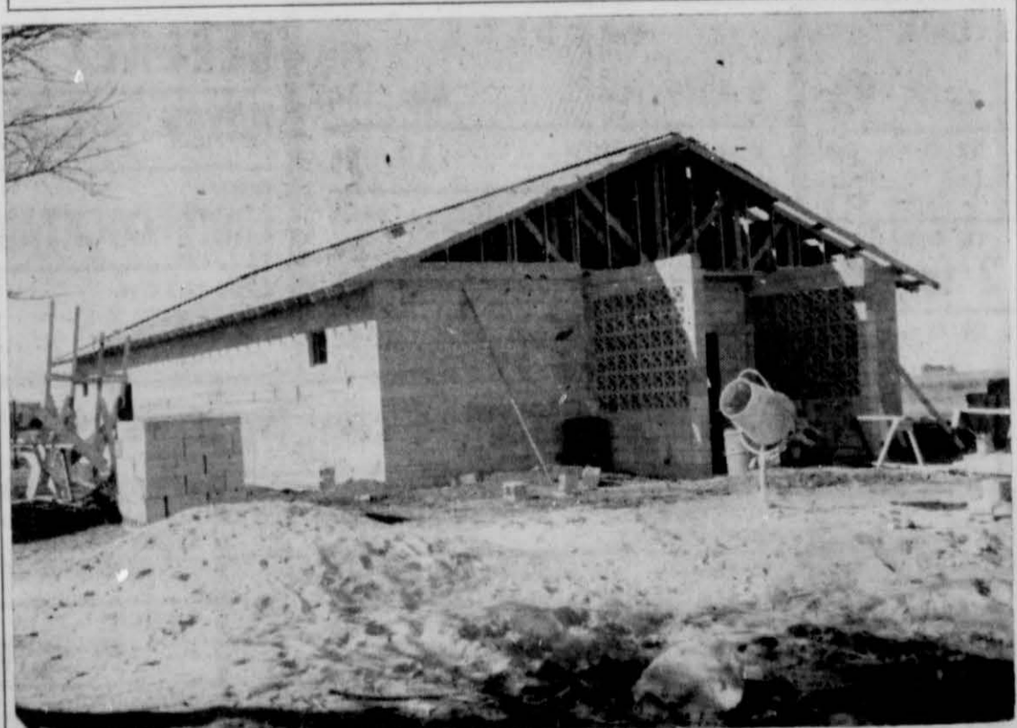
GOING UP —This is the new Northside Baptist Church under construction on West Halsell in North Dimmitt. Virtually all of the work is by volunteer labor from the membership of the church. The concrete block structure measures 36 x 72 feet and will seat 250 persons when completed. Pastor is Rev. Jimmy Gresham, who works on the building, preaches and attends Wayland College in Blaineville. The old church building is behind the new building. —staff photo
