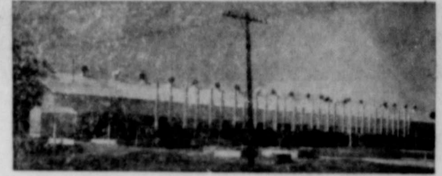
Lone Star Compressor Station No. 3
