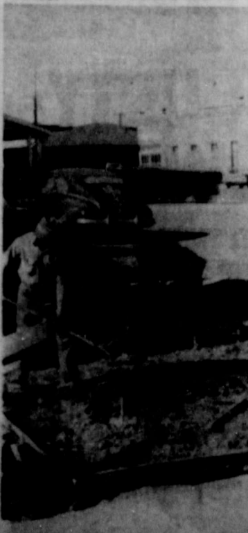
NEW PARKING FACILITIES—Killingsworth Funeral Home is in the process of completing their new parking lot adjacent to the Funeral Home. Workers are pictured working on the new curbing and sidewalks to be installed. The new parking facilities will be completely hot-topped. Bill Bourdeau is contractor for the work. (Photo by Capps Studio)
