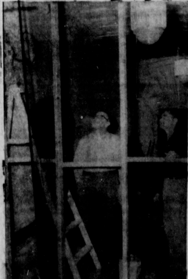
NEW CHAMBER OFFICE —Bill Collings, Roy Plumley, and W. T. Eaton, left to right, are pictured as they work on the new Chamber of Commerce office building. Members of the Chamber are furnishing the labor to renovate the building. (Prints by Capps Studio).
