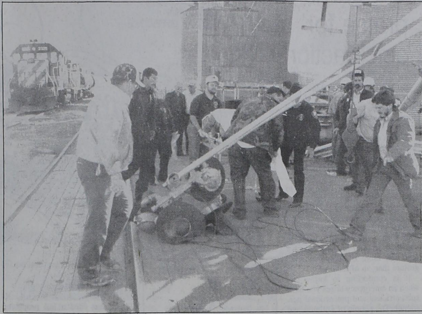
ACCIDENT AT CROSSING INJURES MAN —Local emergency workers tend to injuries sustained by L.E. Carter of Amarillo on Dec. 7 when a crossing signal he was working on collapsed. He was flung from atop the crossing signal onto a beam on the back of a Burlington Northern pickup, then to the pavement. Although he was released after treatment here, Carter was hospitalized later that night in Amarillo for further treatment. The crossing has been blocked since the accident so the signal may be replaced, and for other rehabilitation work as Burlington Northern works to upgrade the local spur. Photo by John Brooks
