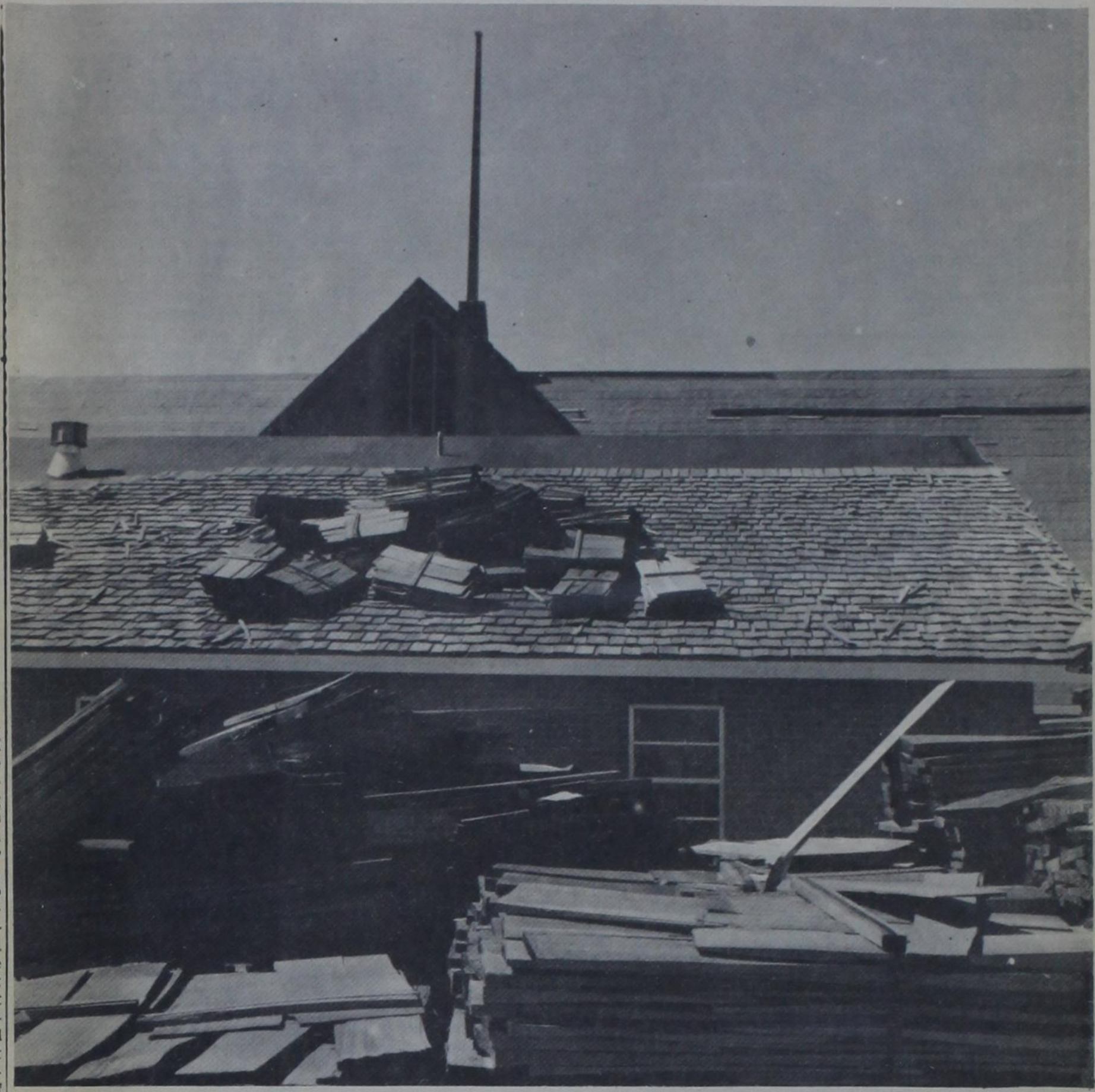
RAISING THE ROOF —It's shingling time at the huge new First Baptist Church construction project. Workmen have tacked down thousands of shingles on the wings of the
