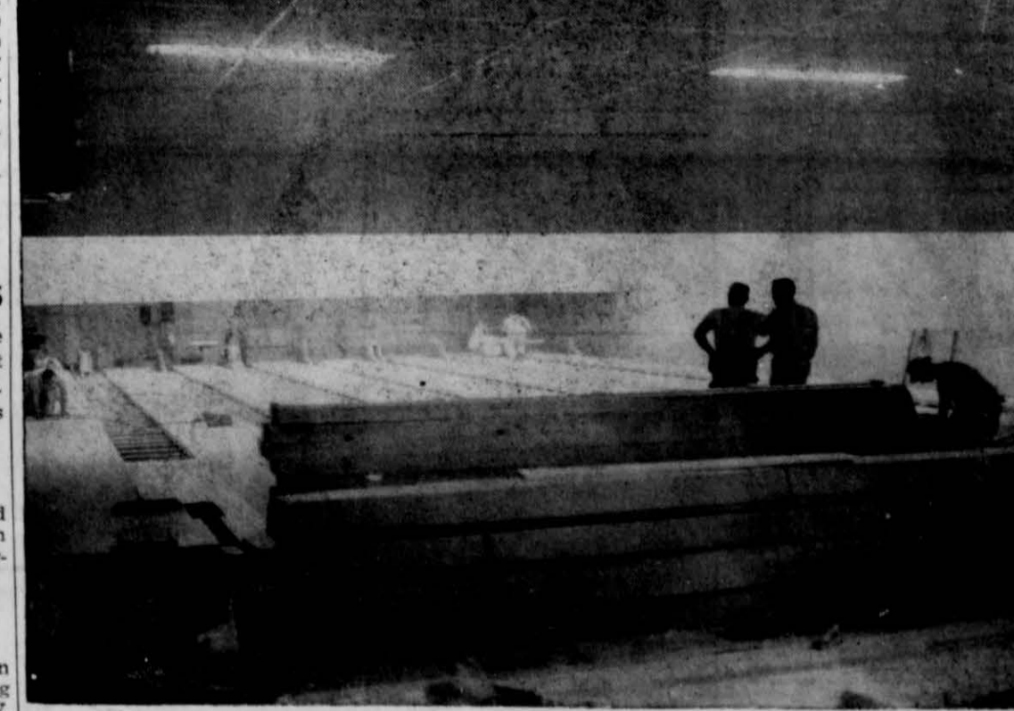
NEARING COMPLETION —The deluxe interior of Cotton Bowl Lanes, Dimmitt's brand-new bowling alley, is nearing completion. Workers are shown here putting down the maple lanes prior to the arrival of the automatic pin spotting mechanisms. Cotton Bowl Lanes will represent the largest single investment in athletic type recreation ever made in Dimmitt. When completed Dimmitt will have one of the most modern bowling alleys in the Panhandle. It will open Wednesday or Thursday. —staff photo
