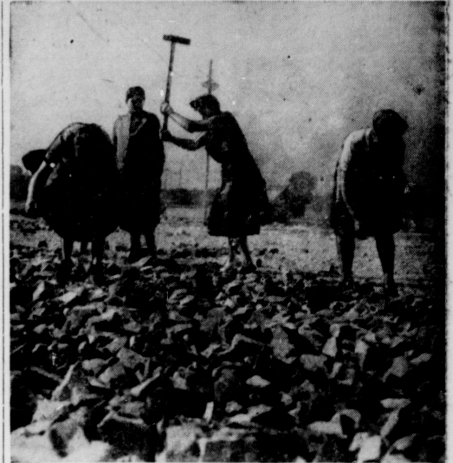
HELP ALLIED AIRLIFT . . . In order to increase the potency and efficiency of the Allied airlift into beleaguered Berlin, more air strips had to be built. Scores of German women, like those pictured above, are aiding the Allies by helping to build a new runway at Tegel, in the heart of the French sector of Berlin. These new strips relieve the heavy burden from the Tempelhof airport.
