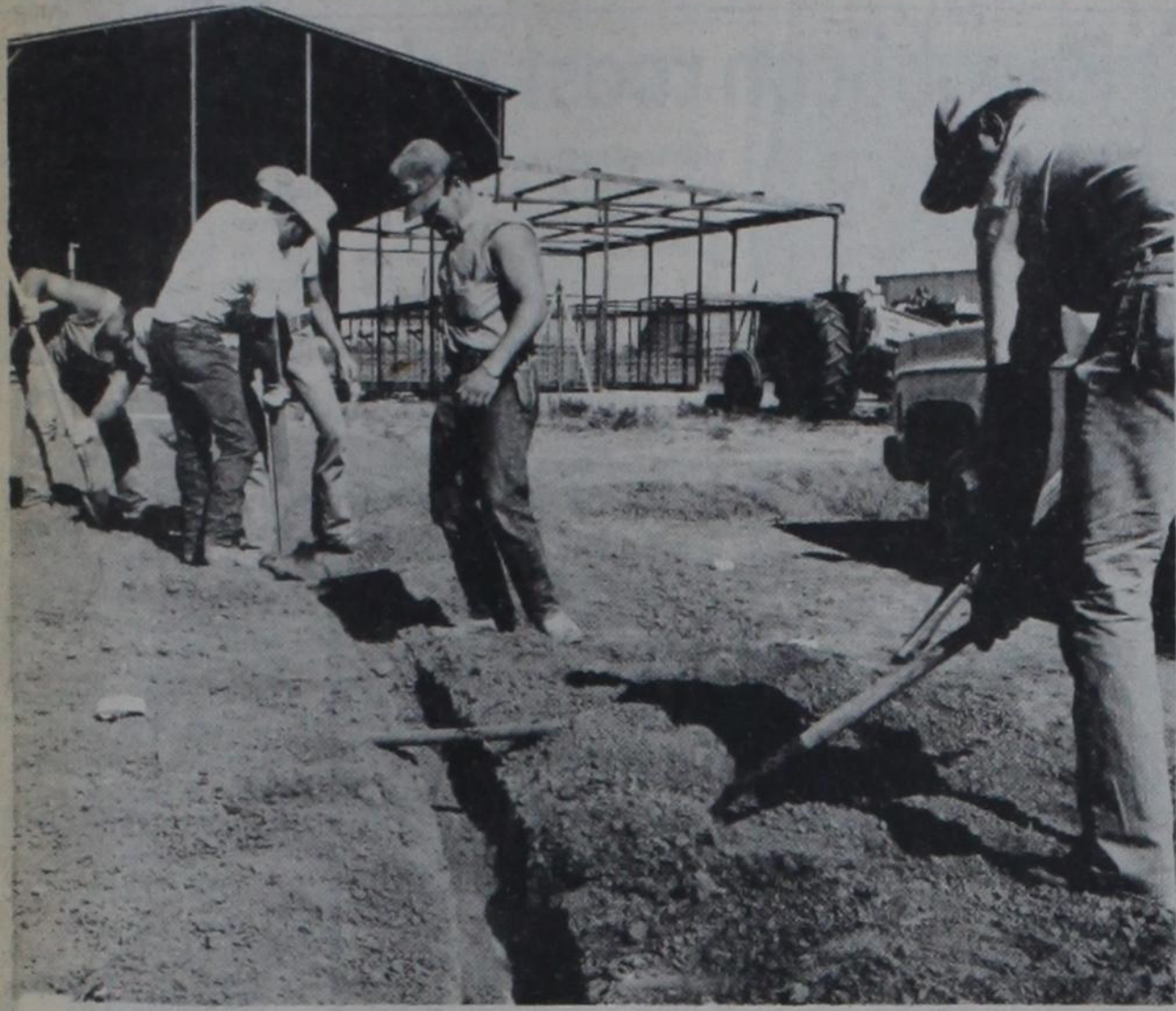
ONE MORE JOB DONE—During a workday at the new FFA Farm south of the airport Saturday, members of the Dimmitt Young Farmers complete work on a drainage pipe from the wash-rack of the work barn. From foreground back are Joe Lust, Dana Wall, Frank Welch, Larry Robb and Randy Schu-
