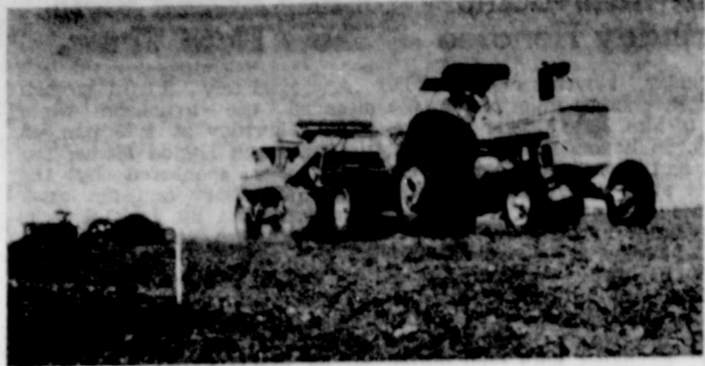
MACHINERY HERE is at work installing a conservation irrigation system on land that was uneven and had too steep of slope to efficiently use irrigation water on the K. E. Probasco place, four miles north of Barwise. Cuts are being made on the upper side with the elevating type buggys and fills made on lower side so a uniform grade of .2 foot falls per 100 feet will be the finished grade. — USDA-SCS photo by J. J. McEntire
