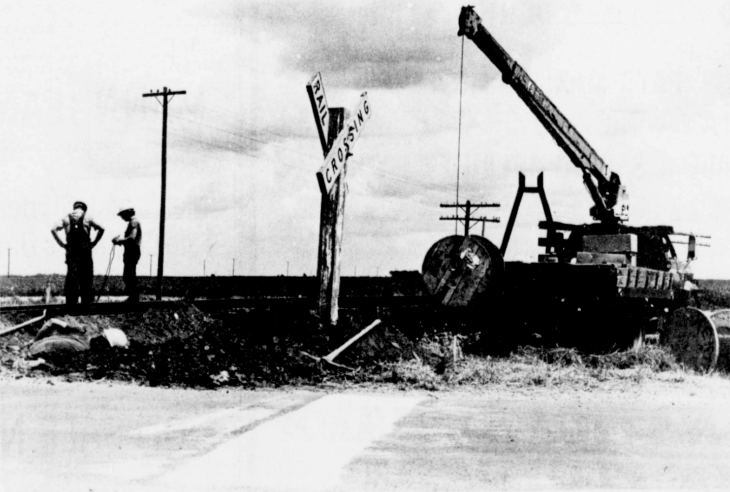
FLASHING LIGHTS and gates are being installed at the railroad crossing where the Santa Fe tracks intersect Farm Road 2301 near Aiken, just north of US 70. Railroad employees are putting in the lights, gates, and sensing devices, under contract from the state. The installation could be complete in two to three weeks. (Staff Photo)
