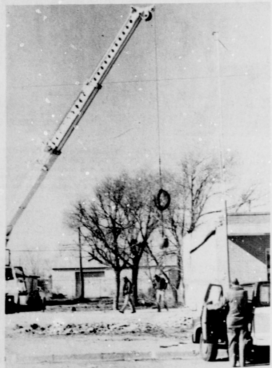
WRECKING CREW — Justice of peace Raz Ford pauses to watch as a heavy steel ball is dropped just a few feet from the side of the building in which his
