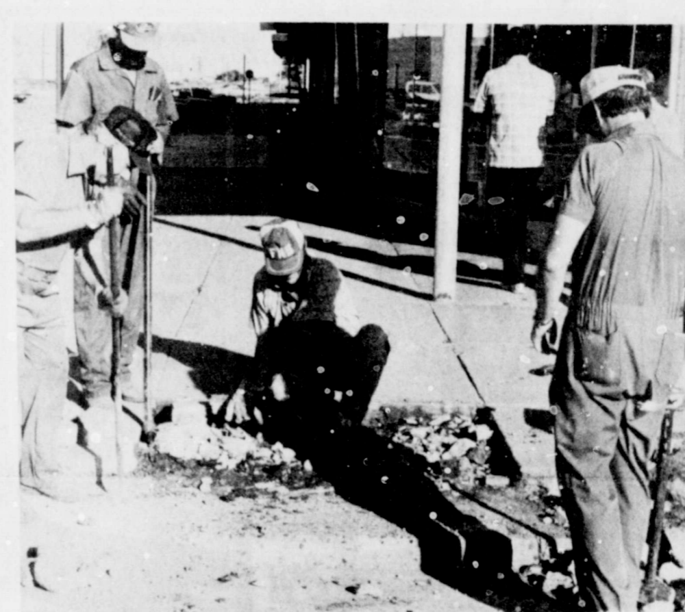
LIONS STARTED BUSTING CONCRETE Thursday. Left to right—Aldine Williams, Bob Aildredge, Gary Brown, Ted Jordan in front of Arwine's Drug Store.
