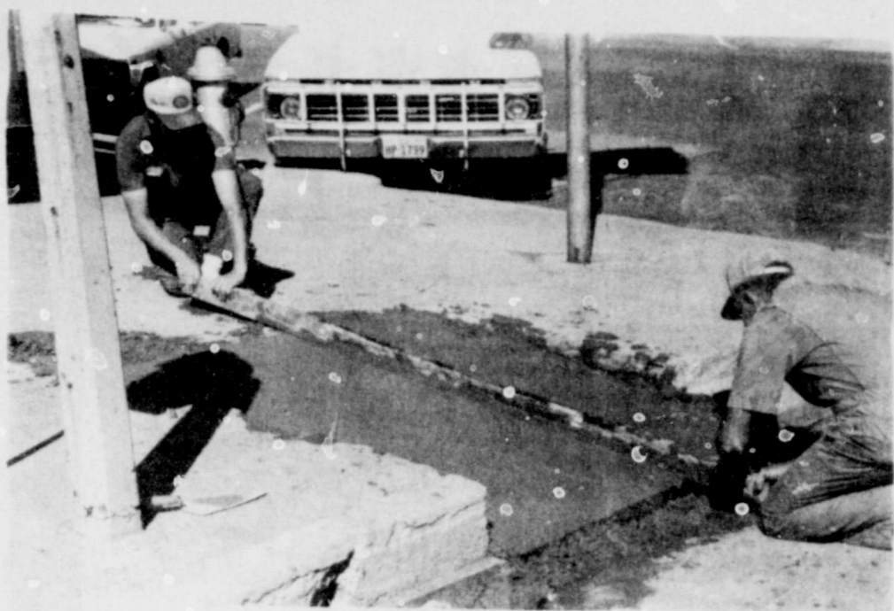
TED JORDAN AND BOB COPELAND are forming the cement in front of Thompson's Pharmacy.
