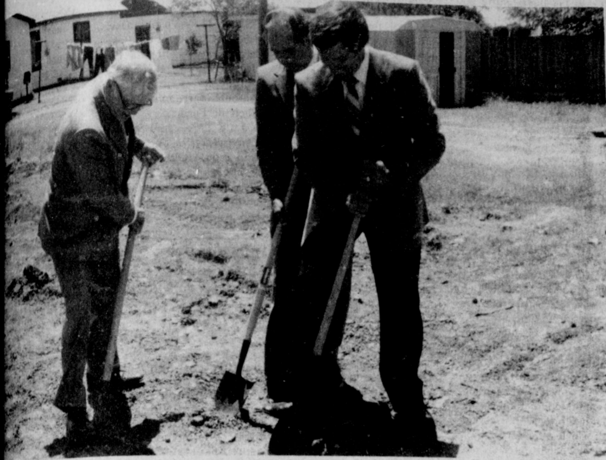
WELL, left, chairman of the Deacons, the Rev. John Jenkins, center, and committee chairman Gail Kring, turned the first shovels full of dirt as ground was broken for the new educational building at First Baptist Church in
