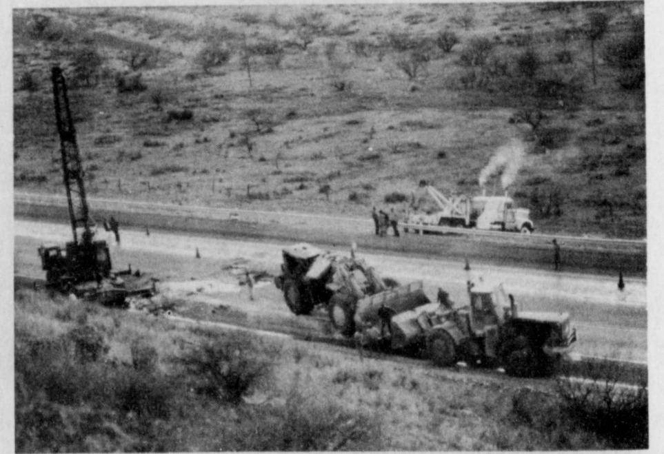
A FRONT END LOADER half the size of the wrecked loader eases the giant piece of equipment down the hill.
