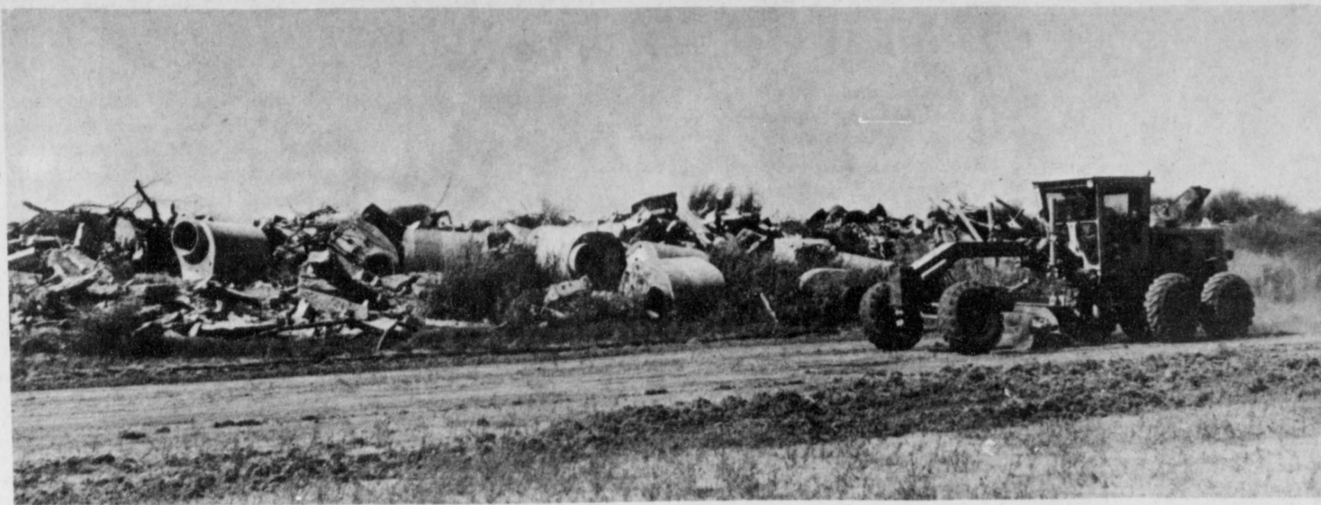
THAT'S A LOT OF CONCRETE TO BURY -- The County Commissioners are digging a new pit at the Lockney dumpground to push the concrete, wire, and old tires into that have been accumulating over the years. The Texas
