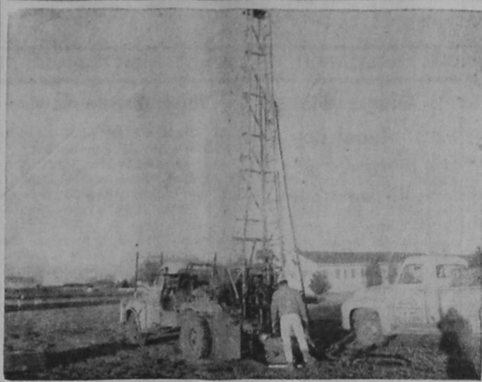
THIS SOIL TESTING EQUIPMENT is used in determining the size and type of foundation for the new hospital which the soil will support. The foundation investigation is being conducted in preparation for the starting of the new County Hospital. J.T. Anderson (kneeling) and Harley Shofner (standing) are technicians for the Texas Testing Laboratories, Inc. in Dallas which will test and evaluate the soil. The laboratory findings will determine the type of foundation necessary for the new building. —Staff Photo
