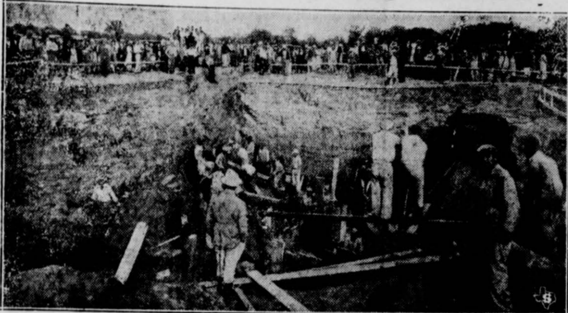
Here is the scene of the cave-in at Bridgeport, Texas, where four men lost their lives. The big hole was a settling basin for the Bridgeport filter plant, under construction. After being buried alive, four workmen were drowned as water came up while their fellow workers were endeavoring to dig them out. The dead are Bud Shawn, 26; Claude Mader, 29; Nolan Gohar, 21 and C. H. Furr, 54. In the picture workers are shown vainly seeking to rescue the four doomed men. (Texas News Photos.)
