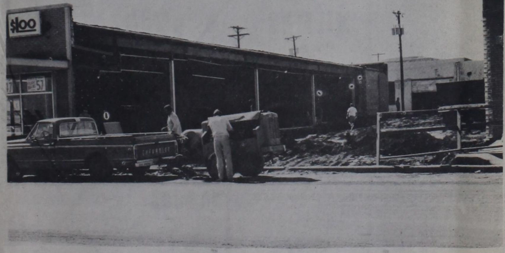
TUMBLING DOWN—The walls and fronts of three stores have come down, and soon new walls will start going up, expanding Dimmitt's TG&Y Store to three times its present size. The expansion project is expected to be completed by mid-year. Note how the original building which houses TG&Y was constructed with steel pillars supporting the weight of the north side, so the wall could be knocked out for future expansion.
