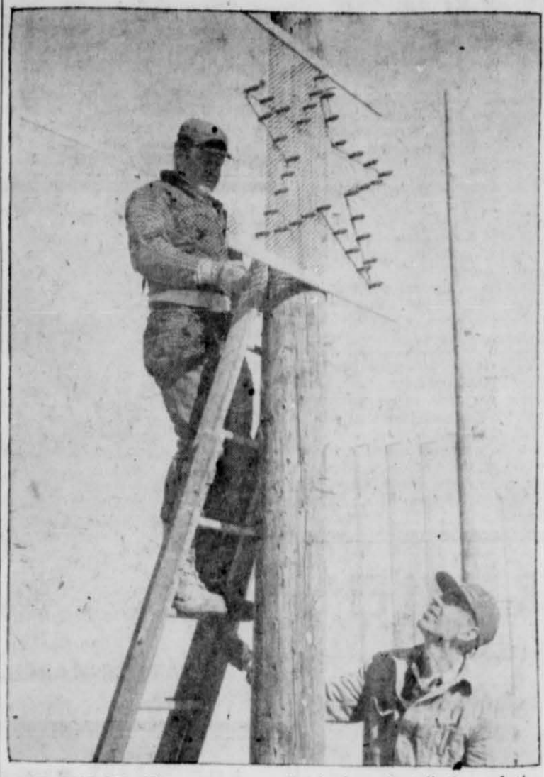
LAST ONE UP —These two men finished up installation of the unique star and tree outline decorations adorning Dimmitt this year's Christmas decorations. They are Lonnie Cork (on ladder) and Buck Raper, both city employees. Workers from many business firms assisted in building and installing the decorations. —staff photo
