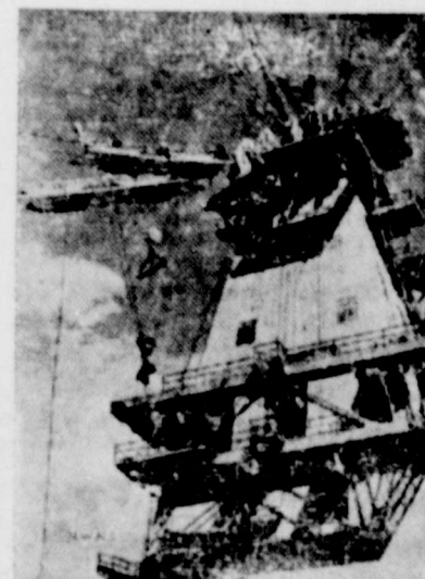
Apex of 460-foot tower built at the Shasta dam on the Sacramento river, California, to aid in the building of the largest concrete dam in the world, with the exception of Boulder. The dam will conserve the water of the Sacramento river for irrigation and power.
