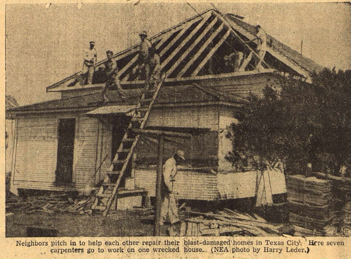
Neighbors pitch in to help each other repair their blast-damaged homes in Texas City. Here seven carpenters go to work on one wrecked house. (NEA photo by Harry Leder.)
