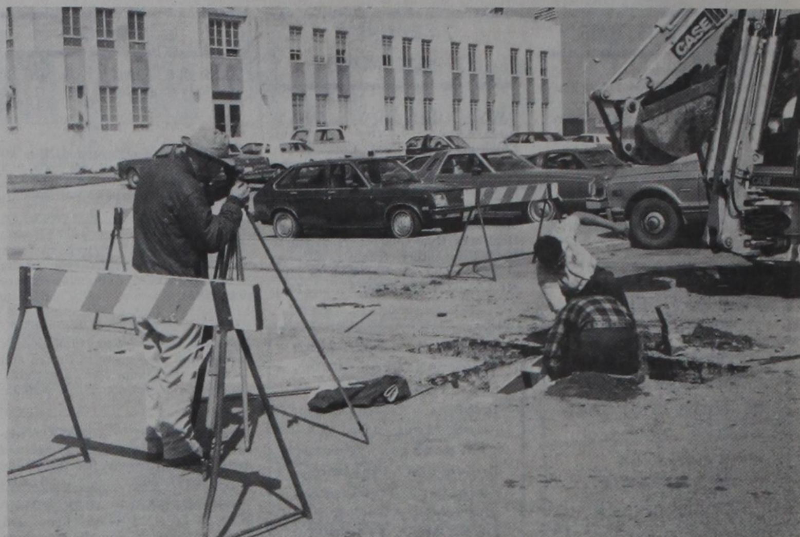
COUNTY SURVEYOR JOHN ALLDREDGE is making sure it's just exactly right, as workers from Dimmitt Ready Mix ready a foundation for a permanent survey marker on the southeast corner of the courthouse square in Dimmitt. The concrete will surround a stainless steel marker, which, with a compa-
