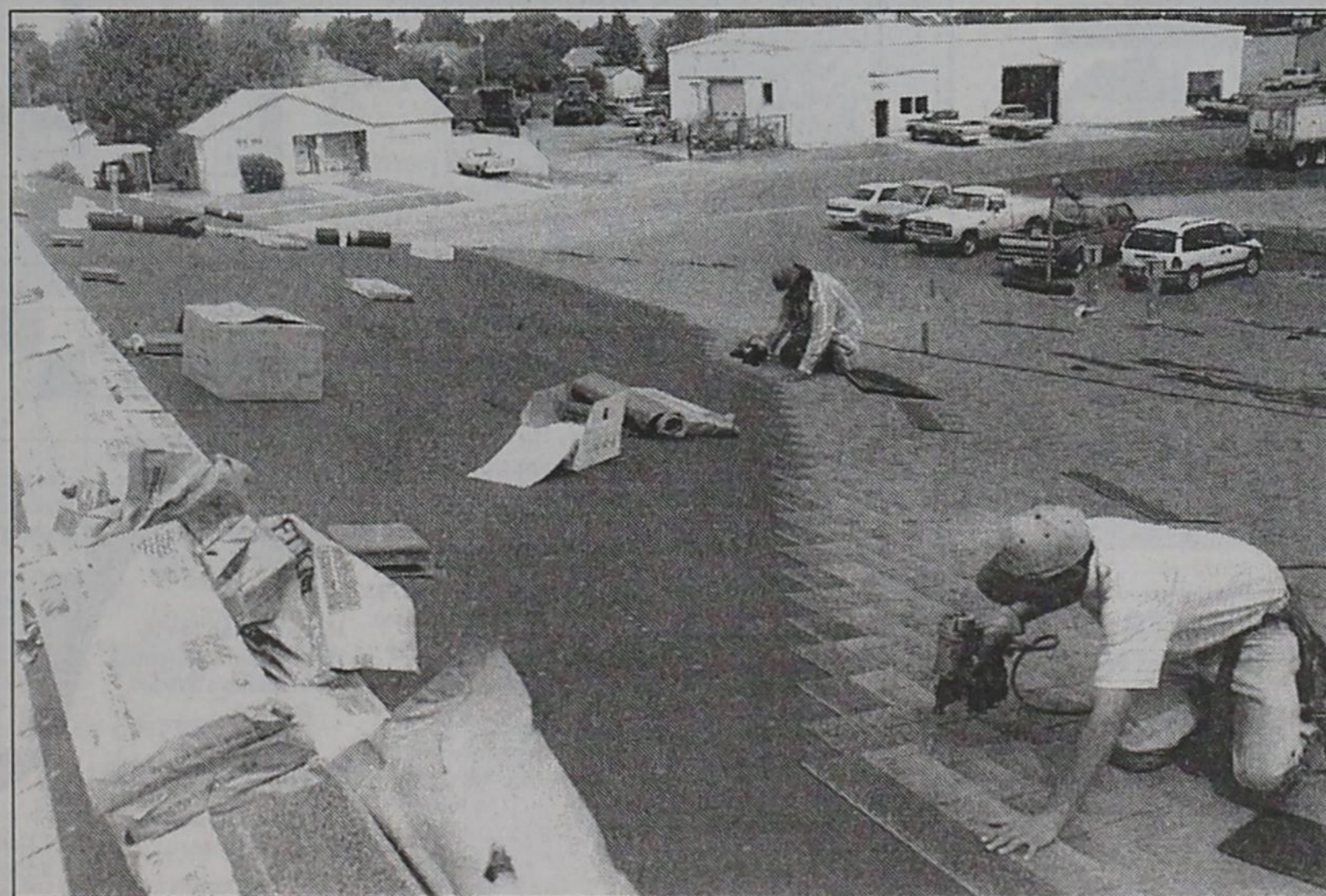
A FAMILIAR SIGHT throughout the county is this one, of roofers working from dawn 'til dusk to repair hail damage on hundreds of homes and businesses. Here, Jesus Miramontes (foreground) of Littlefield
