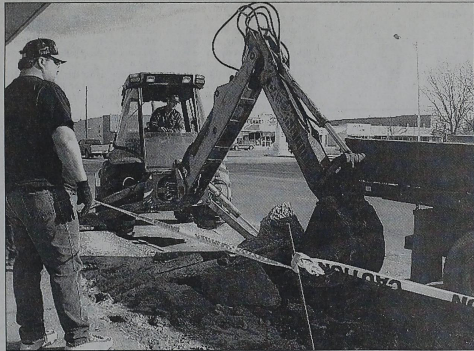
CAN YOU DIG IT?—Raul Jackson watches as Dean Kirby operates a backhoe that is digging up part of the sidewalk in front of Dollar General in Dimmitt
