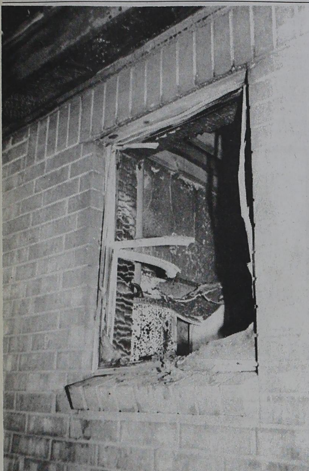
A HOT WATER HEATER barely visible through this window was the culprit in igniting paint thinner fumes that started a fire Saturday evening at 1010 W. Grant in Dimmitt. The utility room of the home was totally damaged. Photo by Don Nelson
