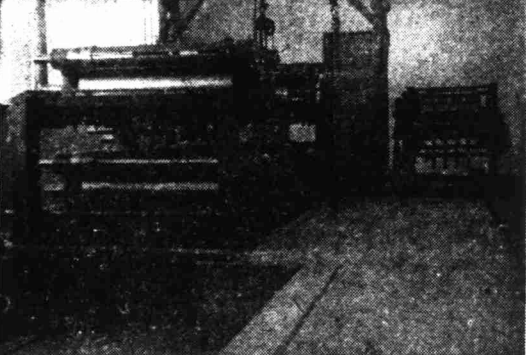
The assembling job progresses as rollers, gears and other parts are installed on the frame. The press was made and assembled in Battle Creek, Mich., where a test run was made. It then was dismantled, the parts numbered, and shipped to Midland for re-assembly in the Reporter-Telegram press room.
