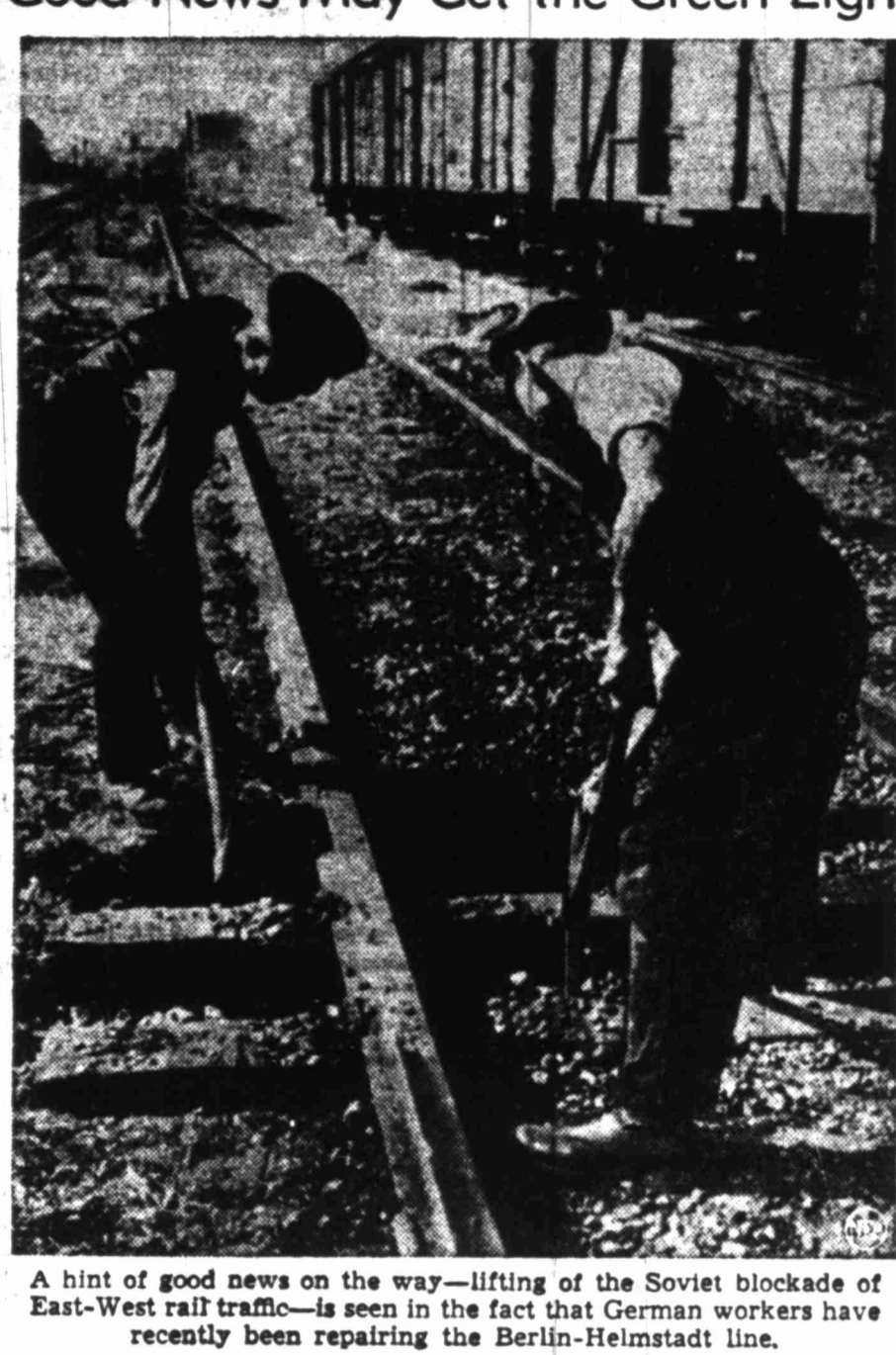
A hint of good news on the way—lifting of the Soviet blockade of East-West rail traffic—is seen in the fact that German workers have recently been repairing the Berlin-Helmstadt line.
