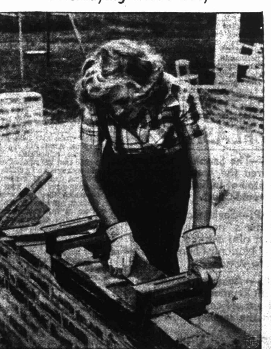
The "first real improvement in five centuries in the method of laying bricks" is demonstrated in Montgomery, Ala., by poed Kitty McGlynn. The device, invented by engineers Paul H. Sommers and John S. Hodgson, is said to speed bricklaying four times the normal pace. Acceptance by the building industry could mean great savings in construction costs—especially in the building of low-cost homes.
