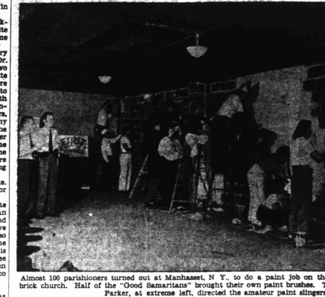
Almost 100 parishioners turned out at Manhasset, N. Y., to do a paint job on the interior of their new brick church. Half of the "Good Samaritans" brought their own paint brushes. The pastor, Rev. George Parker, at center, directed the amateur paint blunders.
