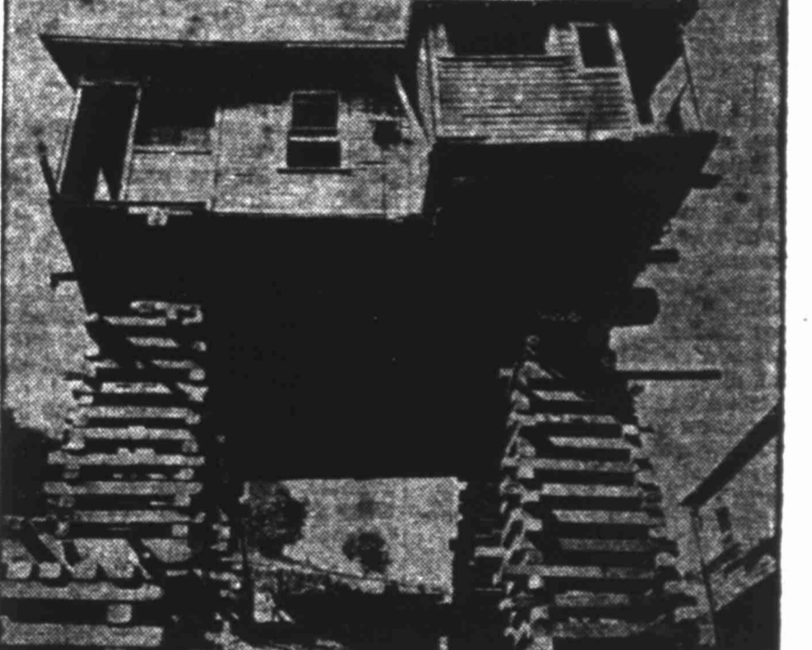
"Watch out for that first step" might well be the warning to visitors to this dwelling near Los Angeles. Construction of a freeway forced removal of the house to a new location; but the place needed a full foundation so workmen propped it up like this until a basement could be dug.
