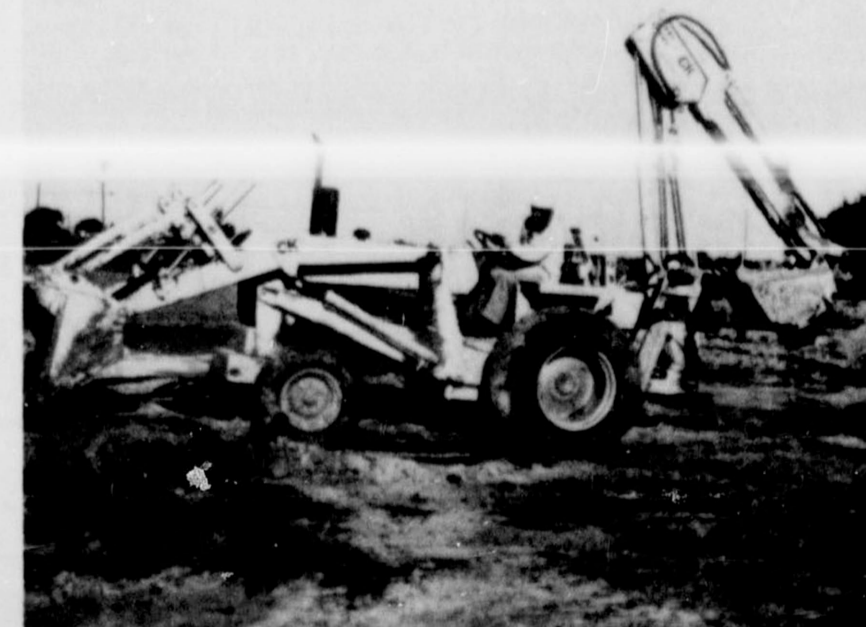
WORK BEGUN...Lewellen Construction Company has begun preliminary dirt work at the Friona
