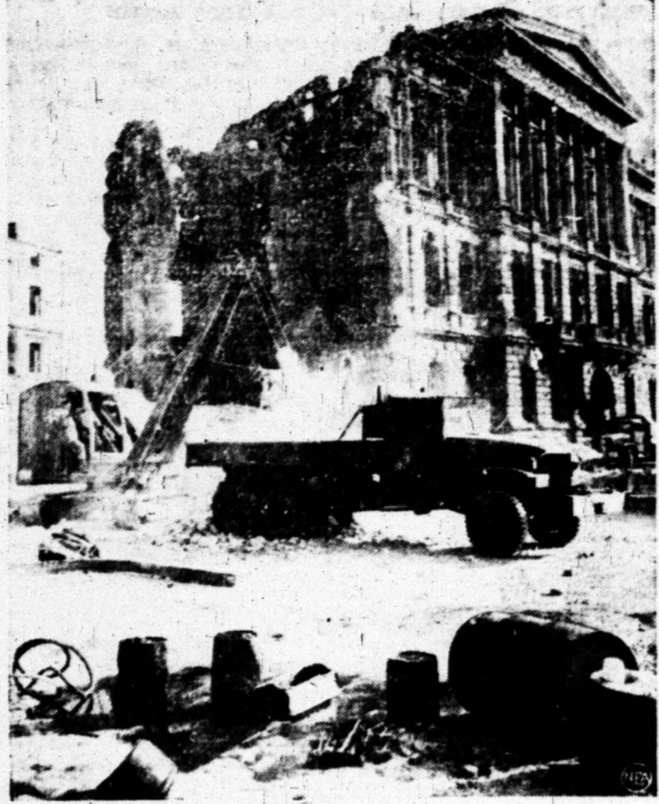
Hit by Allied bombing raids during the war, the U. S. Embassy building in Berlin is just in the process of being cleared. Rubble from the partially destroyed structure is removed by GIs with steam shovels, tractors and trucks. It is thought that many records may still be intact in the embassy basement. (Photo by NEA-Agnes staff correspondent Al Cocking.)
