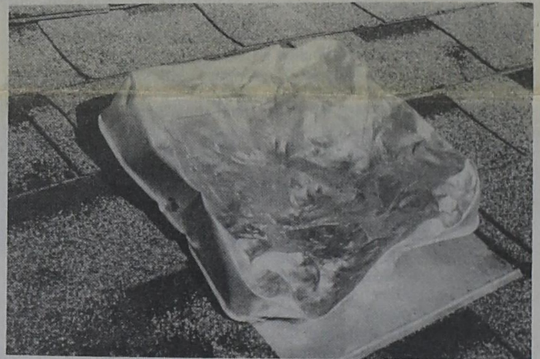
BENT VENT....This attic vent, located on top of Mark Gammon's residence, shows the severity of the hail that fell last week destroying roof tops, windows and crops.
