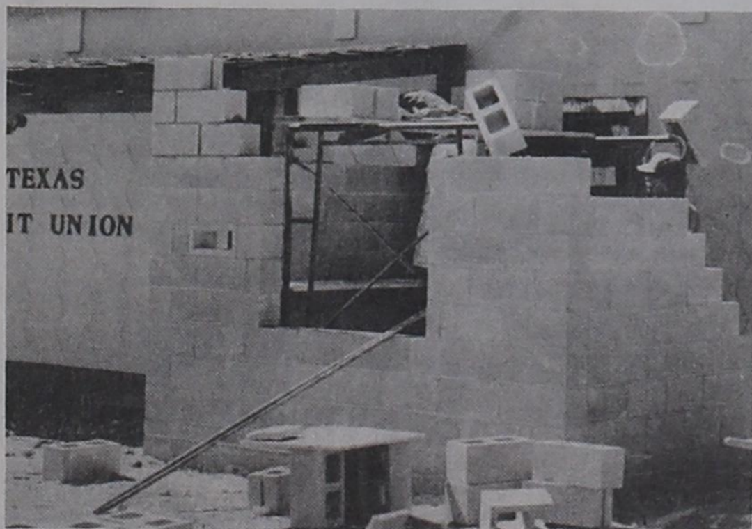
NEW CONSTRUCTION....A new drive-up window is being added to the local Credit Union, as part of a remodeling project taking place.
