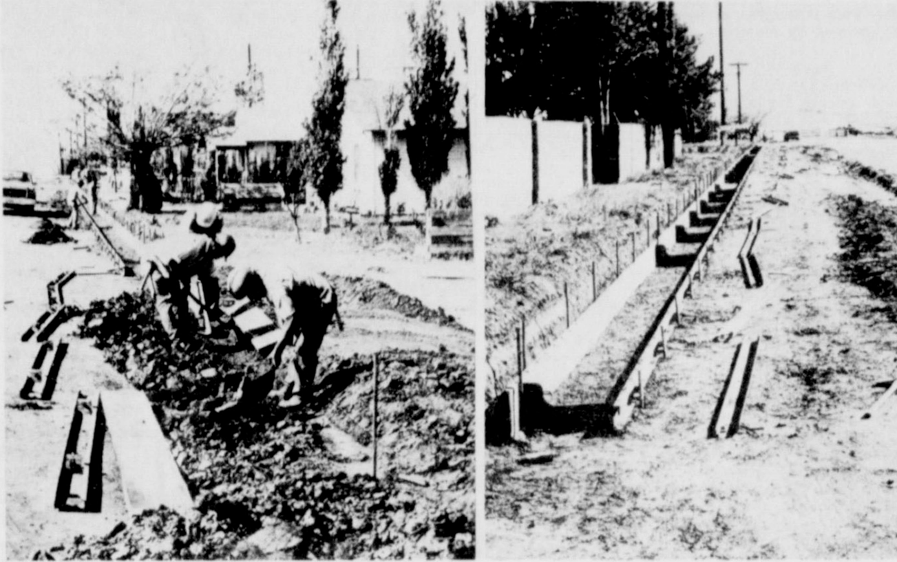
STREET WIDENED....Work to widen Grand Street, which is an extension of Highway 214, began last week, and workmen are shown placing forms for the new curb and gutter along the east and west sides of the street. Warm weather has helped keep the highway and overpass project moving at a good pace in recent weeks.
