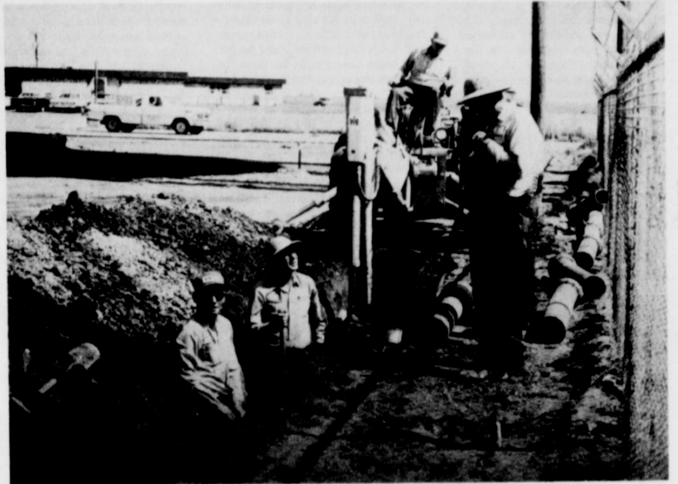
WORK COMPLETED....City of Friona employees completed a one block extension of the city sewer main line to furnish service for the new Senior Citizen House of Friendship
