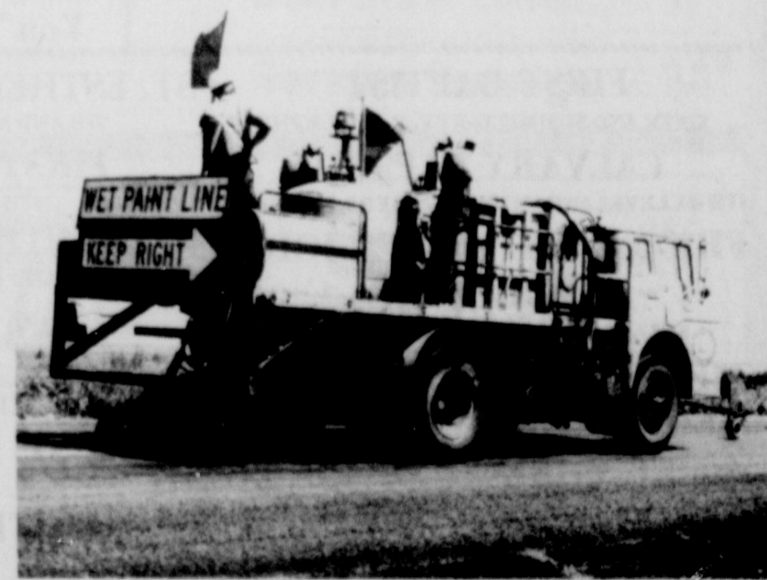
LANE ADDED....The Department of Highways & Transportation crew and equipment are shown painting the stripe for the new left turn lanes, at the east and west approaches to
