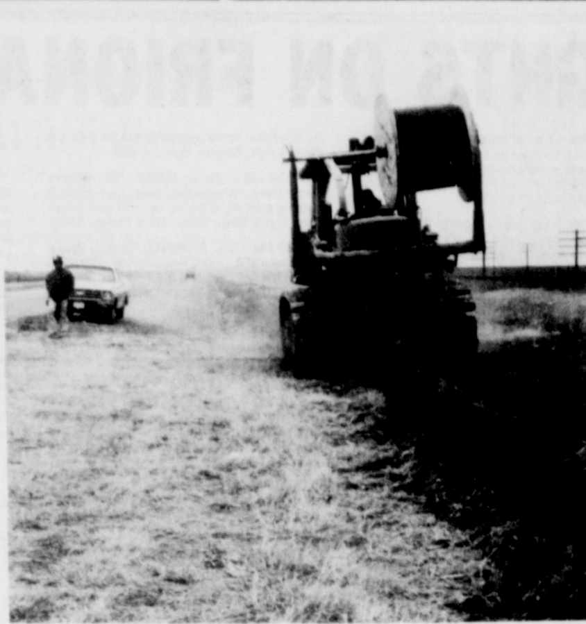
CABLE WORK.... Work was progressing this week on the new underground telephone cable being laid between Bovina and Friona. The new cable, which will replace overhead lines which have been in service since 1920, improve long distance service between the two cities.
