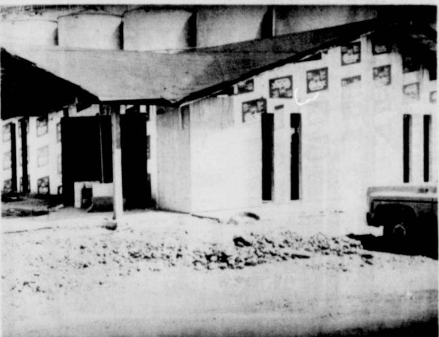
NEW BUILDING....The new office for Friona Wheat Growers Cooperative is beginning to take shape on South Main Street in Friona. This is one example of several building projects underway in Friona this summer.
