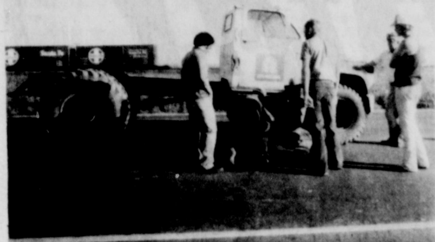
WORKER KILLED.... An employee of Borsberry Construction Co. was killed Monday on the road construction job just west of Friona on Highway 60. Patrolman Art Lopez is shown with others at the scene.
