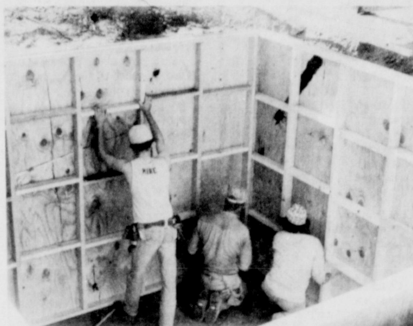
DIGGING IN.... The new building which is going in next door to the Friona Star on Main Street will be the new Friona Cablevision office quarters. Work is currently being done on a basement for the building with much activity from heavy equipment in the area.
