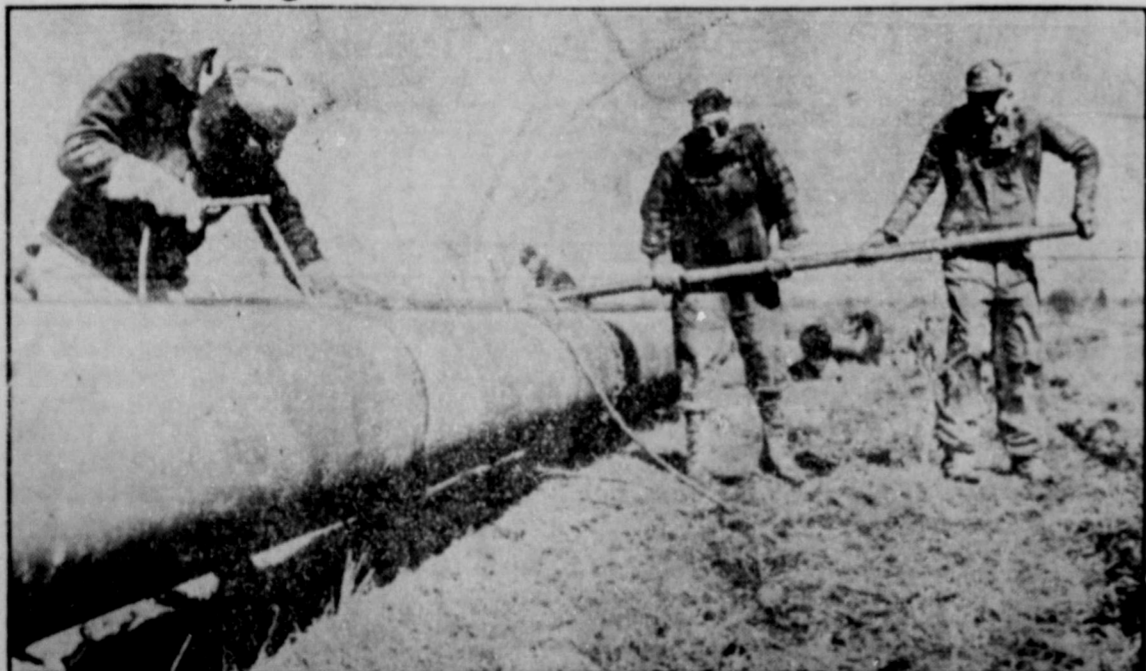
Welders at Lambertville, N. J., connect the long, long iron snake through which oil will flow from Texas to the oil-famished east coast.
