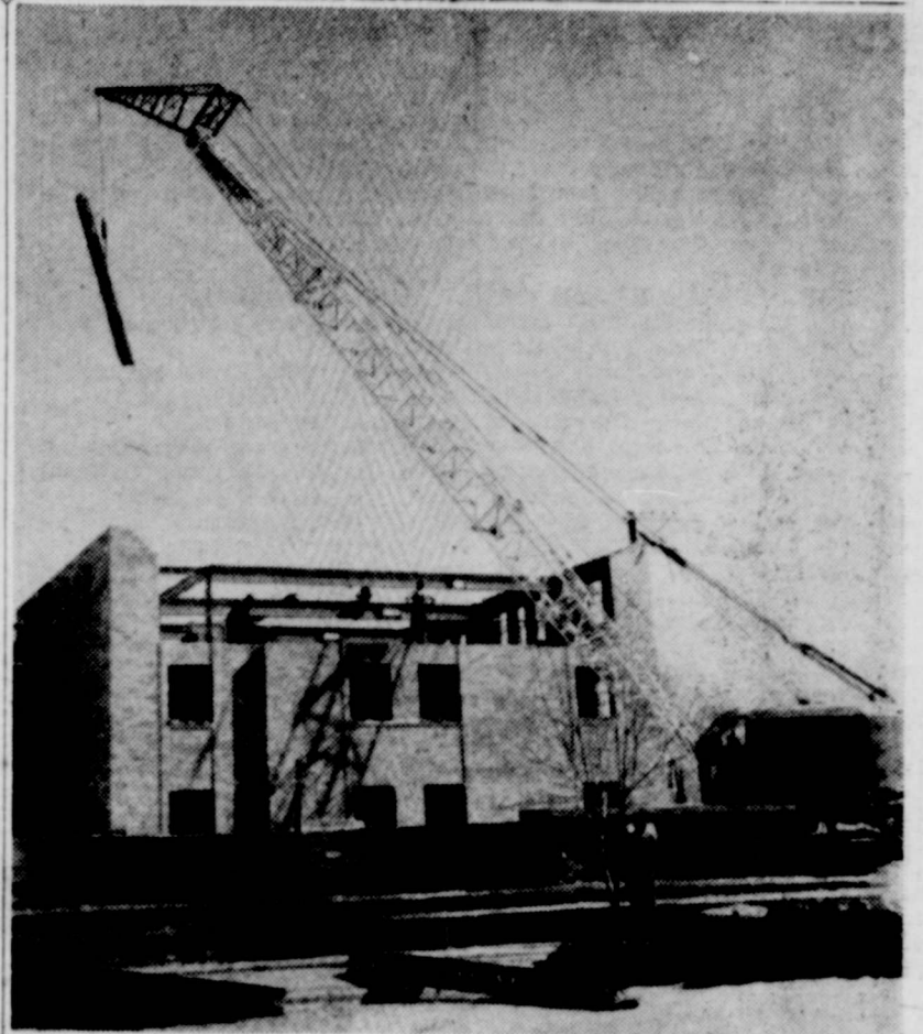
Third Floor Steel was hoisted last week-end as the First Baptist church educational unit continued to go up on South Main street, adjacent to the church auditorium. The giant machine of the Irwin brothers, steel erectors, lifted the last piece of steel into place Thursday. Present prospect is that the unit will be finished ready for occupancy about May 15.
