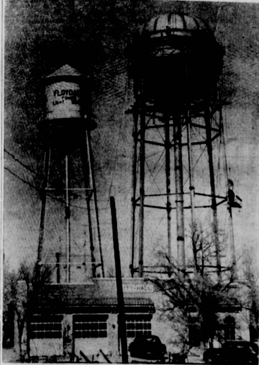
New Sky-Line The environs of the city hall has a new look in the sky-line. The new elevated storage tank standing adjacent to the old, nears completion as the tiny-appearing men crawl over its surface giving it final touches before inspection, the final test and the painter. The bottom of the new tank is higher than the full water level in the old. The city put nearly five times as much money in the ground as the big tank represents in the expansion of the sewer and water system.
