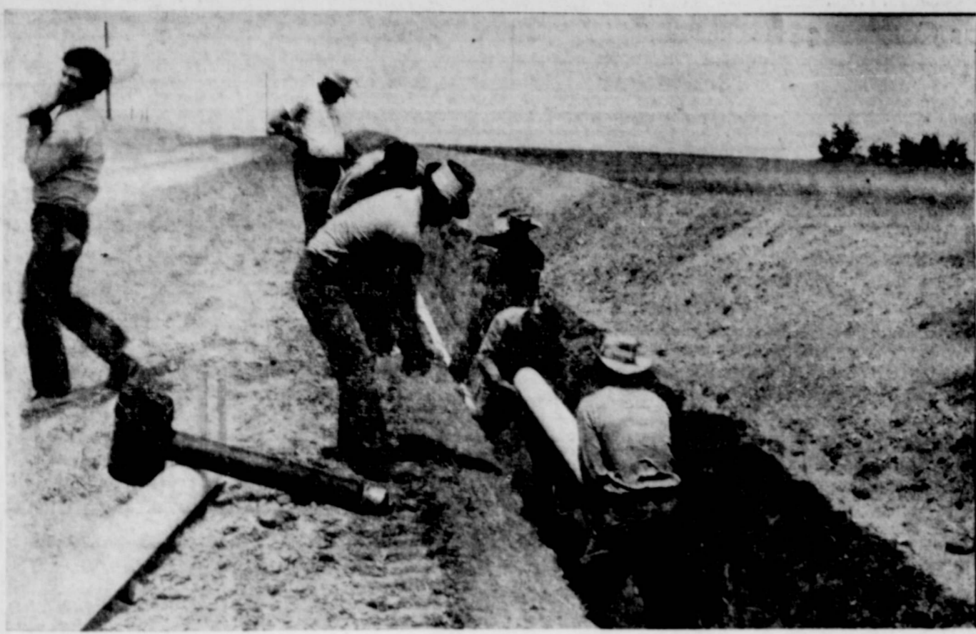
Installation of high pressure irrigation line for sprinkler irrigation system on the Leroy Durham farm west of Sandhill store. Joints are 6" asbestos-cement and designed to stand pressures up to 75 pounds. Installation being installed by Gifford-Hill Western crew out of Lubbock, Texas.
